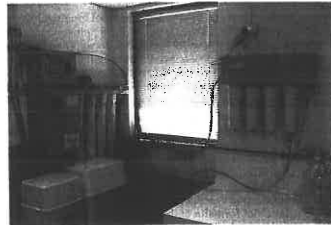
Fig. 9.1 Water purification system showing pre-filters, water softener and carbon filter prior to reverse osmosis (double unit) followed by deionization and ultrafiltration.
